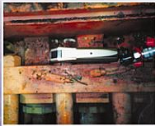
TX-4 With Hex Reducer Working Corroded Fasteners Off-Shore
