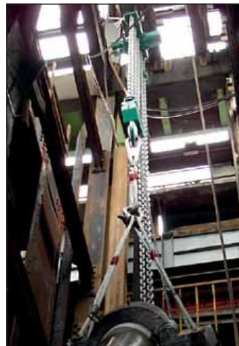
JDN Air Hoist PROFI 37TI mounting a pipe string in a shaft. At the end of this work the PROFI hoist has to position a 1000m long string with a total weight of 30ton.
