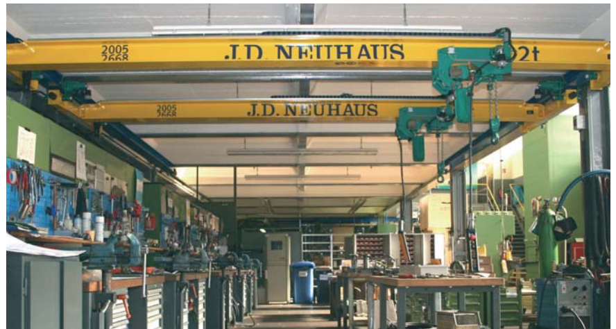
JDN Underslung Cranes with low headroom trolley in an assembly shop.
