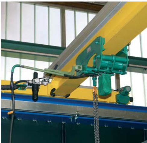
JDN Monorail Crane with control at extension arm.
