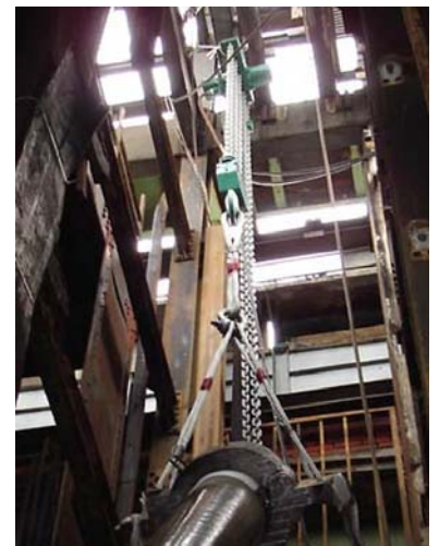
JDN Air Hoist Profi 37 T1 mounting a pipe string in a shaft. At the end of this work the Profi has to position a 1000 m long string with a total weight of 30 t.
